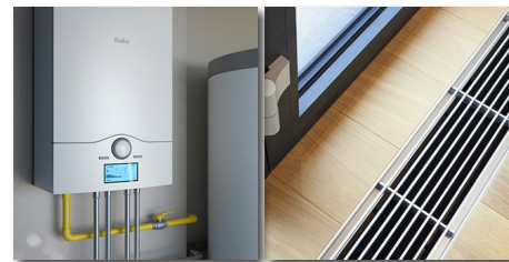
Water heater automation
